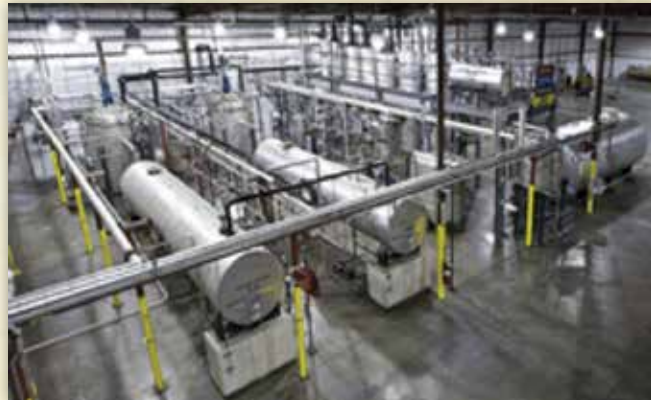
Figure 1.5 Integrity Biofuels – Central Indiana's first soy biodiesel fuel production facility
